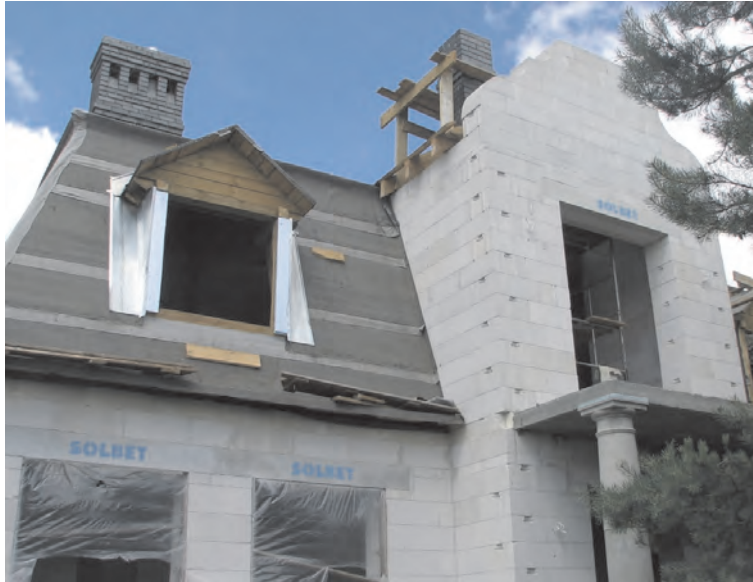
Photo 1. Single-family building of ACC construction, system-based project by a small construction company
