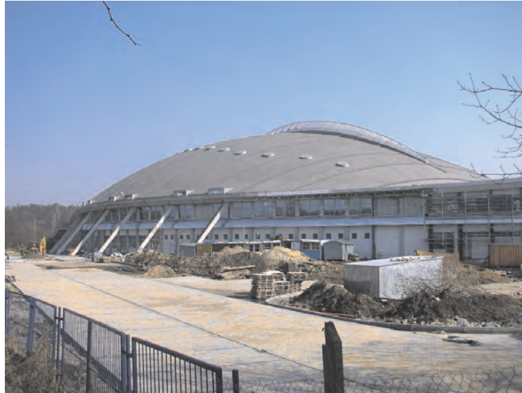
Photo 8. Cycling track building in Pruszków. Reinforced concrete structured filled with ACC wall elements
